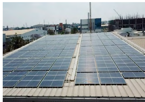
Shindengen India solar power generation system
